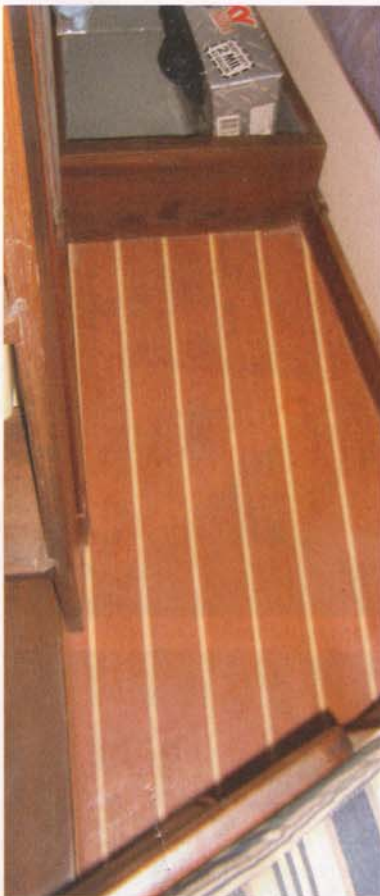
A section of the new flooring after the job was finished. The Degrasses' meticulous approach yielded a boat that looked brand new below.
